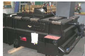
Transformer with bio-degradable oil
